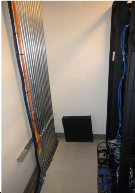
Clear space behind equipment racks
