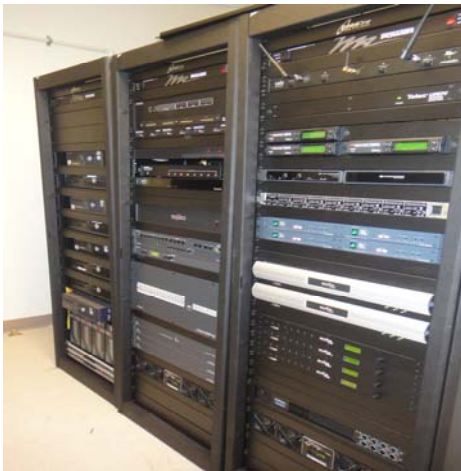
Typical Contemporary AudioVisual Equipment Room
