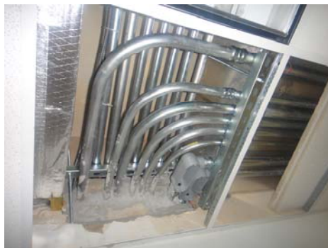
AudioVisual EMT near Equipment Room
