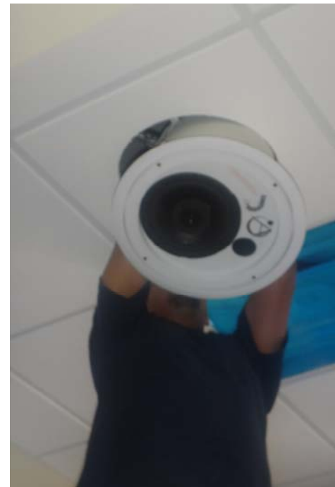
Self-contained loudspeaker solution being installed in an "old work" ceiling. Pre-planned clearance above is critical
