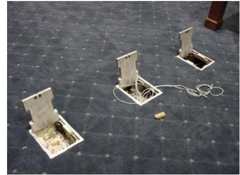
Multiple Unattractive Access Points in a Trench-Duct Floor to Provide Fast Access
