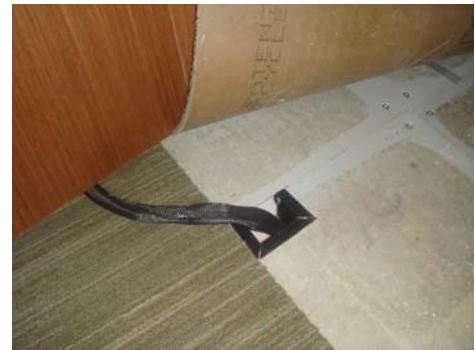
A "mousehole" at the edge of a floor tile. Also, note how the carpet tile overlaps the intersection of four floor tiles.
