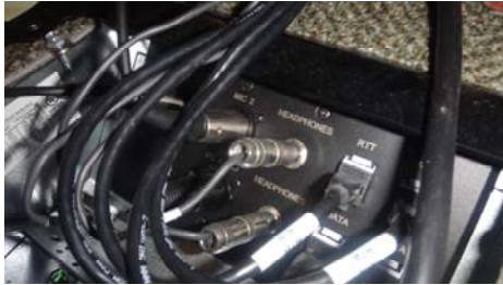
Floor box that is below the finished floor and suitable for AudioVisual use
