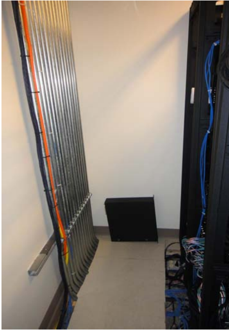
Clear space needed behind equipment racks for access
